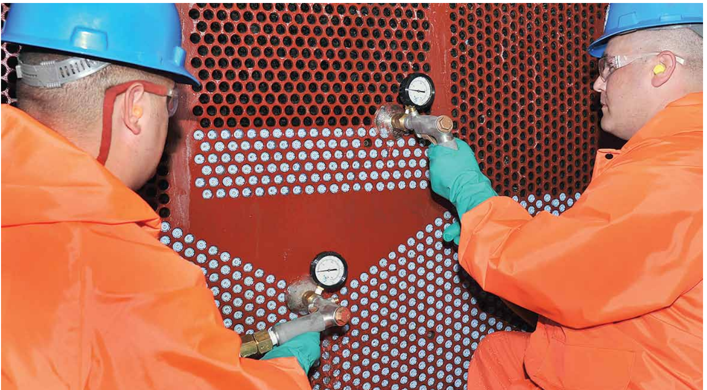
The photographs on this page show examples of Conco tube cleaning projects. Upper photo: small condenser, big deposits. Lower photo: low-pressure mechanical tube cleaning underway
