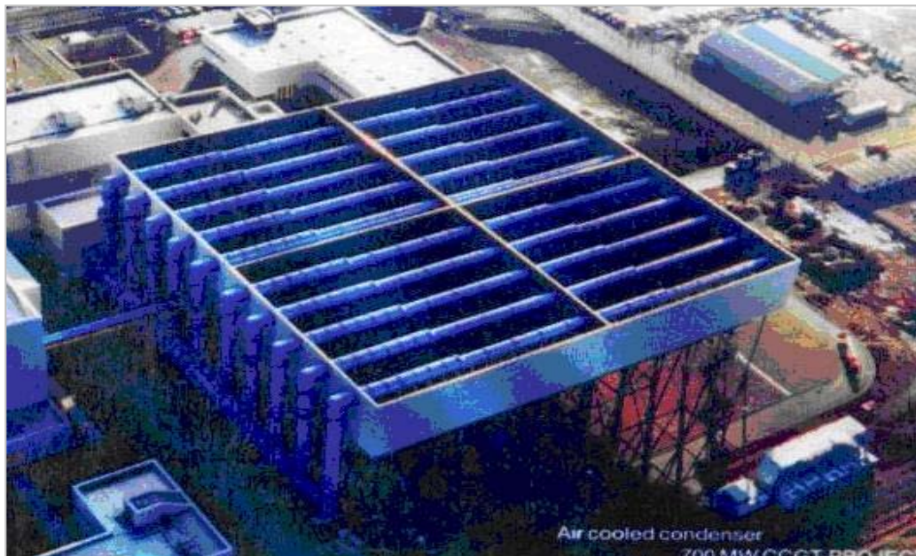
These Air-Cooled Condensers at this 700MW power plant are routinely cleaned with the Conco FinTech™ Cleaning System.
