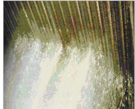
Water is jetting out of the bottom side of a finned ACC during cleaning because nozzles have an optimum angle to ensure spray all the way through the tube rows
